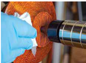
The layup epoxies, West Systems, System 3, or equivalents can be brushed on, applied with rollers, or by hand with a towel
